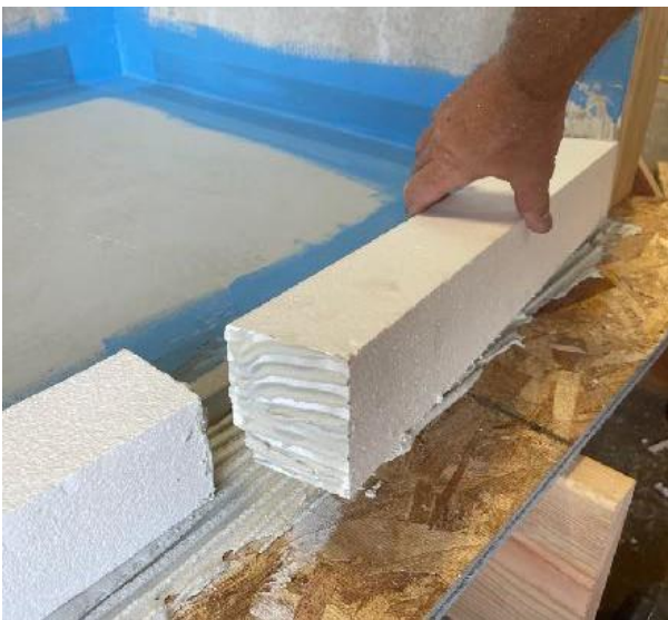
Keeping the curb elevated enough to avoid thin-set contact at the base is good practice
