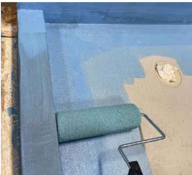
When tanking the shower, the perimeter tape can be coated using a roller (as shown) or a 4" brush
