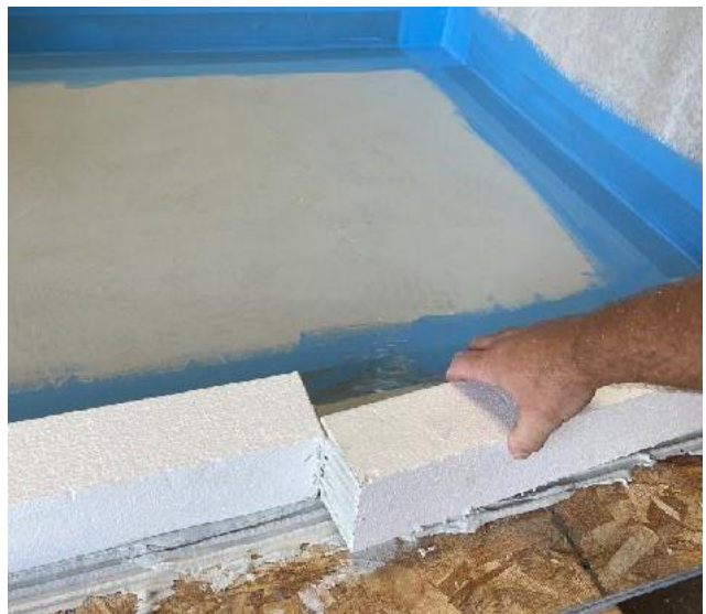
Keep pressure on the curbs towards the outside walls to avoid losing too much thin-set when sliding the second curb in to meet the first one
