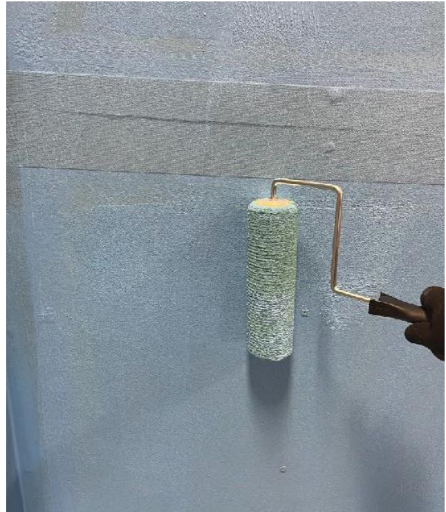
The second coat will be applied in the opposite direction (90 degrees) as the first coat
