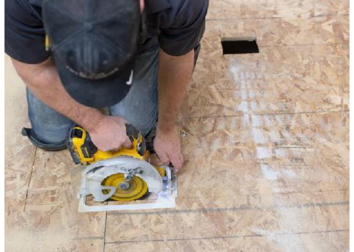
Set saw blade depth to the thickness of the subfloor and cut along traced lines
