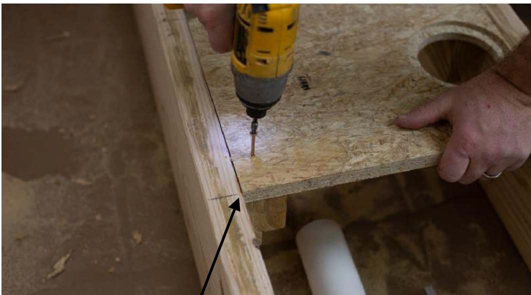
Line drain support block up with traced lines on joist then fasten to drain support block cleats
