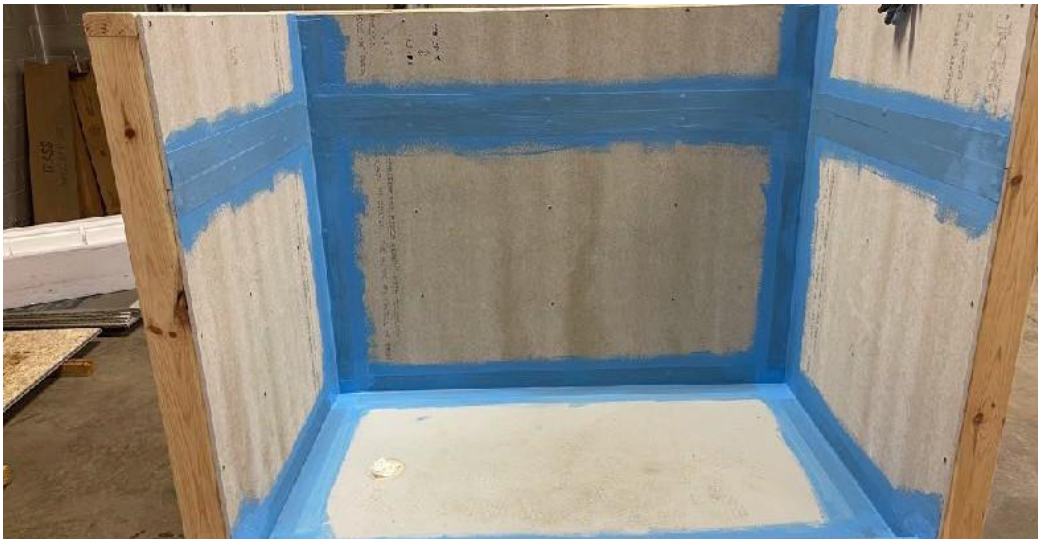
Once all joint tape is embedded you may immediately begin sealing the shower with a 3/8" nap roller
